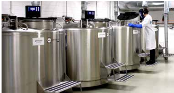
Liquid nitrogen storage tanks - FIMM/University of Helsinki, Finland
